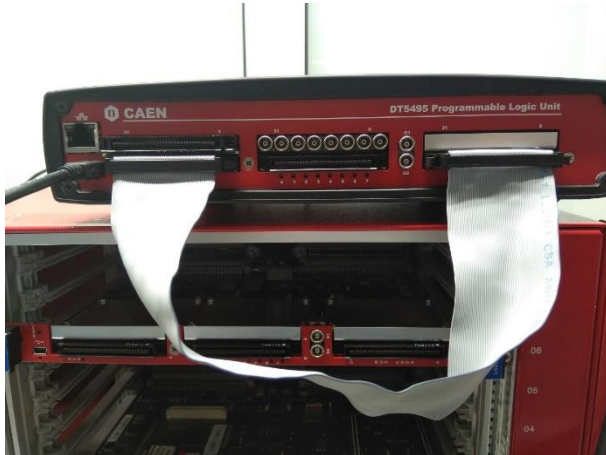
Fig. 7.1: A and C ports of the DT5495 shortcircuited by a Robinson-Robinson cable
